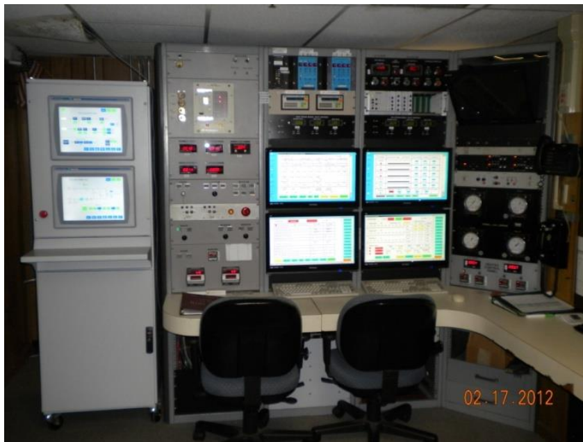
Figure B-2 LSAWT Control Room, CJES standalone console on the left.
